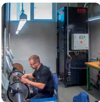
DUSTOMAT Hydro wet separator in the grinding shop
