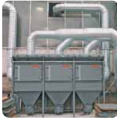
Modular filtration unit
