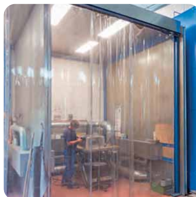
Wet separators are installed on the four grinding booths to safely separate the partially explosive dust
