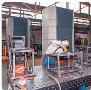
Two filter towers ensure clean air in the welding shop
