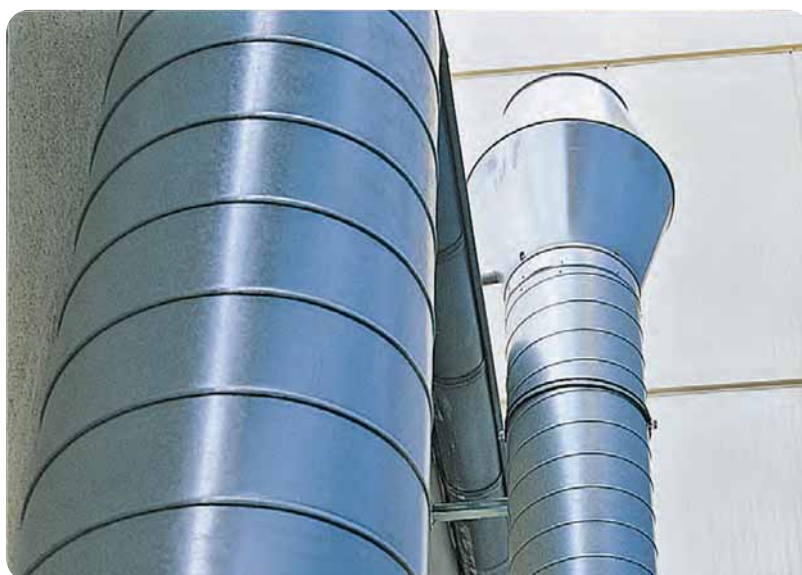
Extract air pipe with deflector hood
