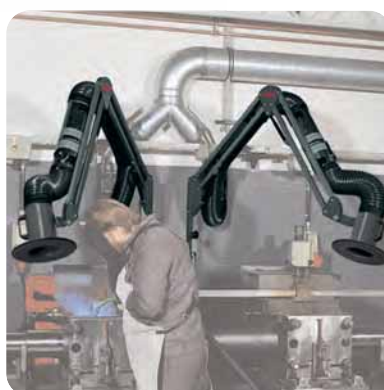
Extraction arm at a welding station
