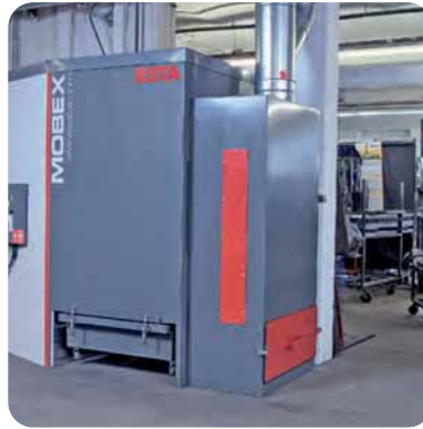
MOBEX F-60 in the production hall
