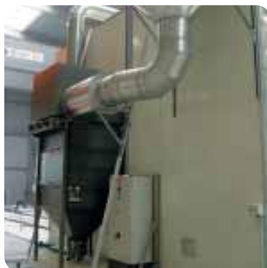
DUSTMAC filter unit on sanding station
