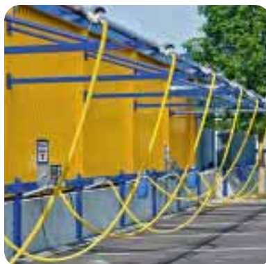
A rigid pipe installation connects the vacuum locations with the cyclonic filter
