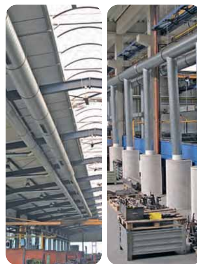
ESTA Upstream Stratification Ventilation
